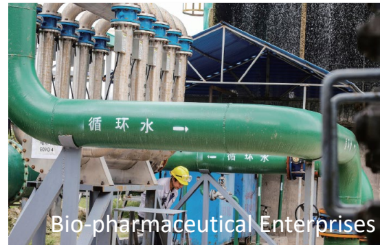
Industrial water circulating
